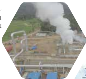
EPC For Geothermal Power Plant
