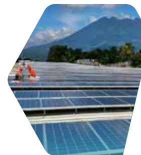
EPC Solar PV Project in Ciherang
